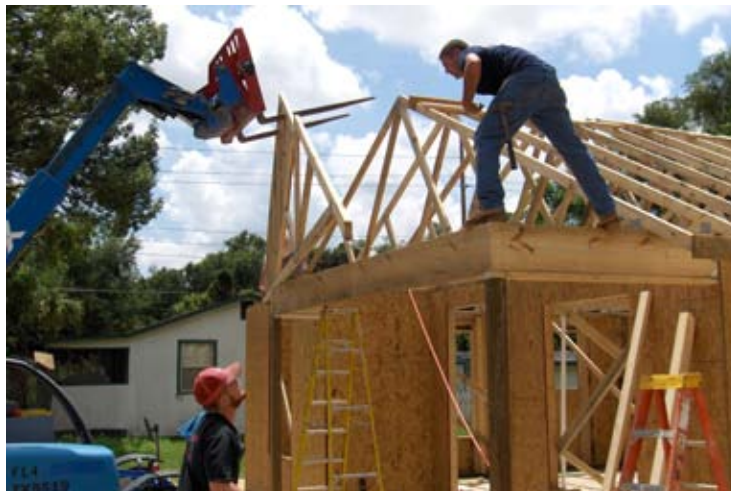
Volunteers from Freedom Fire secure the trusses on the roof of the Ezell house the weekend after Tropical Storm Faye.
